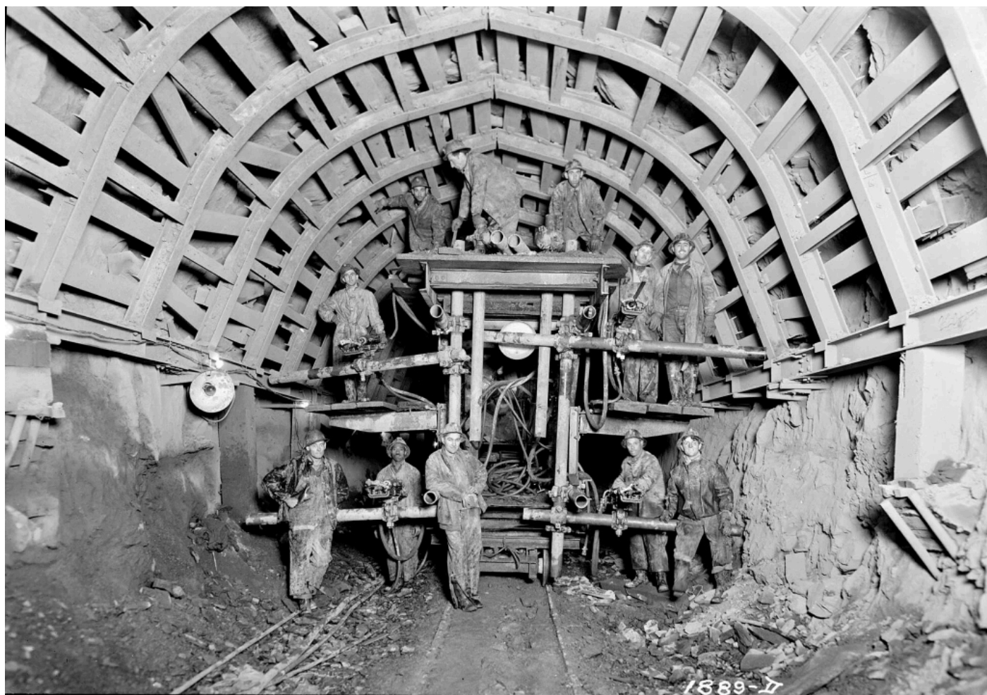
Workers with a drill carriage in the Rondout-West Branch Tunnel, a part of the Delaware Aqueduct. Photo taken October 24, 1939, during the construction of the aqueduct. Source: NYC DEP archives .
